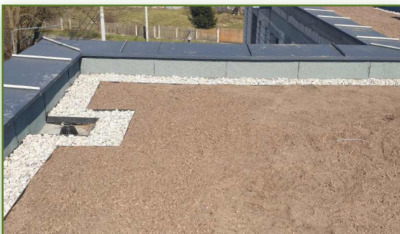
5. The gravel strip has to be approx. 20-30 cm wide and should run along attics, skylights, and inlets
